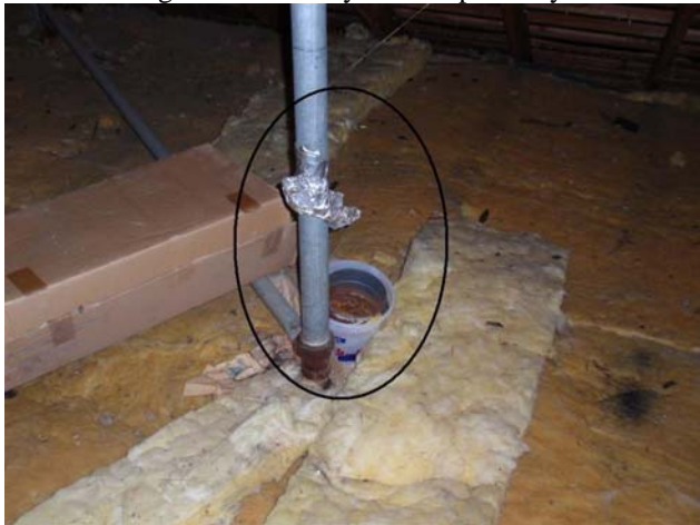
Left over from a leak years ago. Removed bucket
